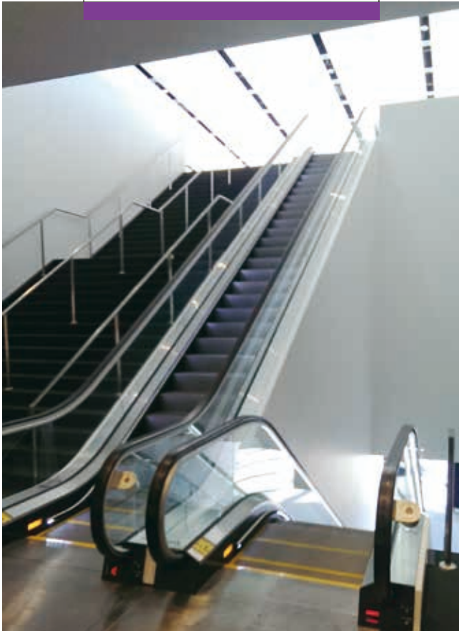
Owensboro Convention Center, USA This multi-purpose convention centre in downtown Owensboro along the Ohio River is western Kentucky's premier meeting space. Anlev has provided escalator units.
